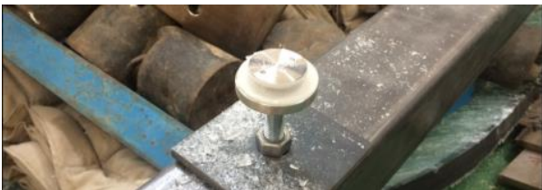
Fig. 18: The steel elements along with the threaded bars stayed on the places
