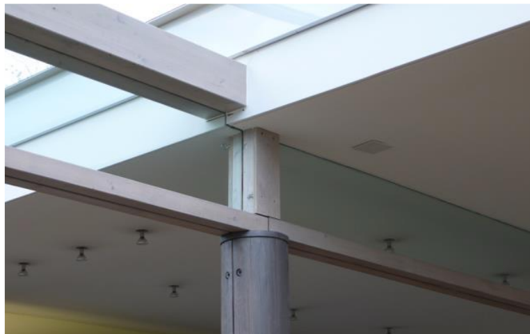
Fig. 2: Photo of the TGC beam at the Palafitte Hotel in Monruz, Switzerland (courtesy of J. Natterer)
