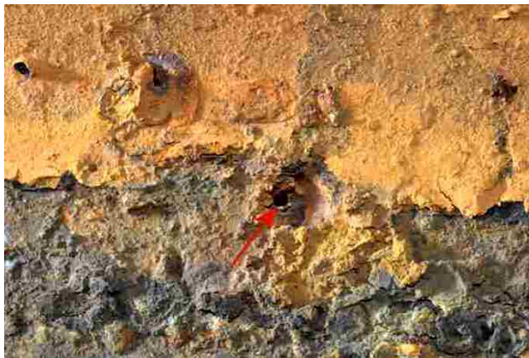
Fig. 3: High Corrosion in Steel portable water cylinder
