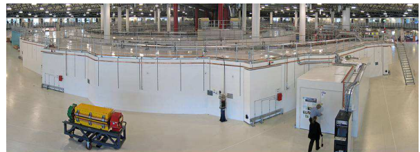
Fig. 23: The interior of the Australian Synchrotron facility. Dominating the image is the storage ring, showing the optical diagnostic beamline at front right. In the middle of the storage ring is the booster synchrotron and linac
