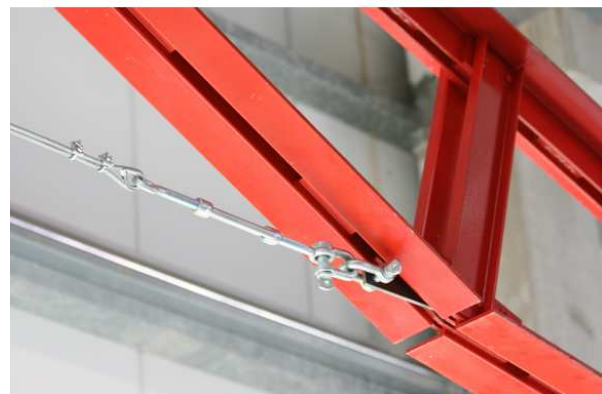
Fig. 7. Built-up members in the roof girder of a temporary GFRP structure (Dicuonzo et al. , 2012)
